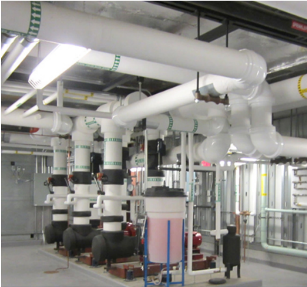
CHILLED WATER SYSTEM
