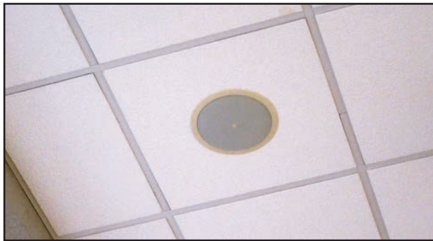
Figure 14.50 A recessed voice evacuation system. Courtesy of Rich Mahaney.
