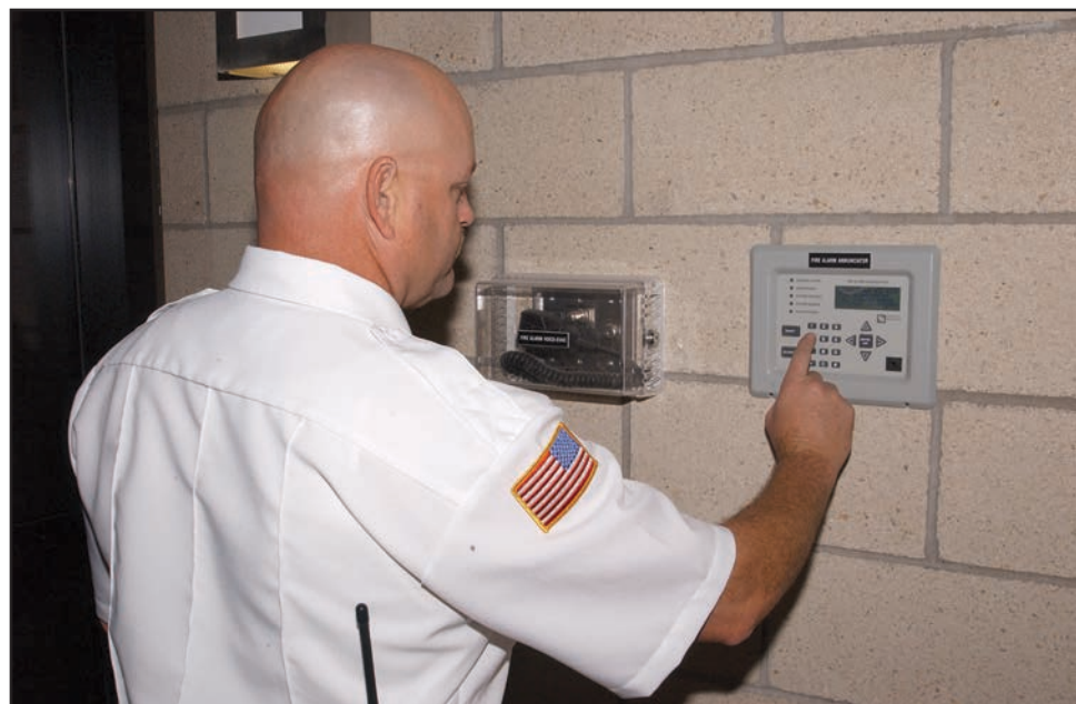
Figure 14.44 Inspectors must verify that all the switches and detector lights on annunciator panels work when tested.
