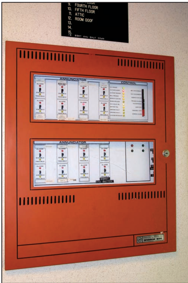
Figure 14.3 An FACU can monitor alarms, control elevators, and public address messages.
