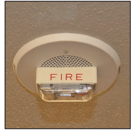
Figure 14.6 A ceiling-mounted fire alarm speaker and strobe light combination unit.
