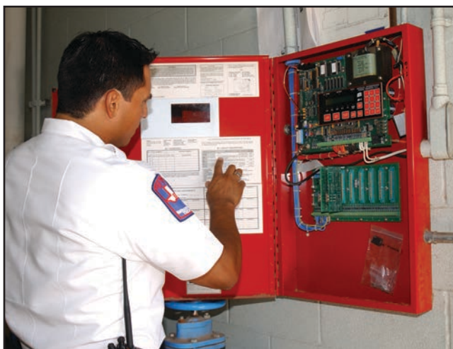
Figure 14.47 Verify that the circuitry and wiring match the system drawing.
