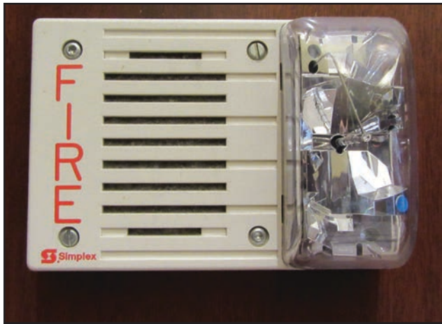
Figure 14.49 Verify that occupant notification devices are consistent with the requirements of the locally adopted code. Courtesy of Rich Mahaney.
