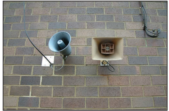
Figure 14.19 One-way voice communication systems are commonly used to provide occupants in a structure with instructions during an emergency.
