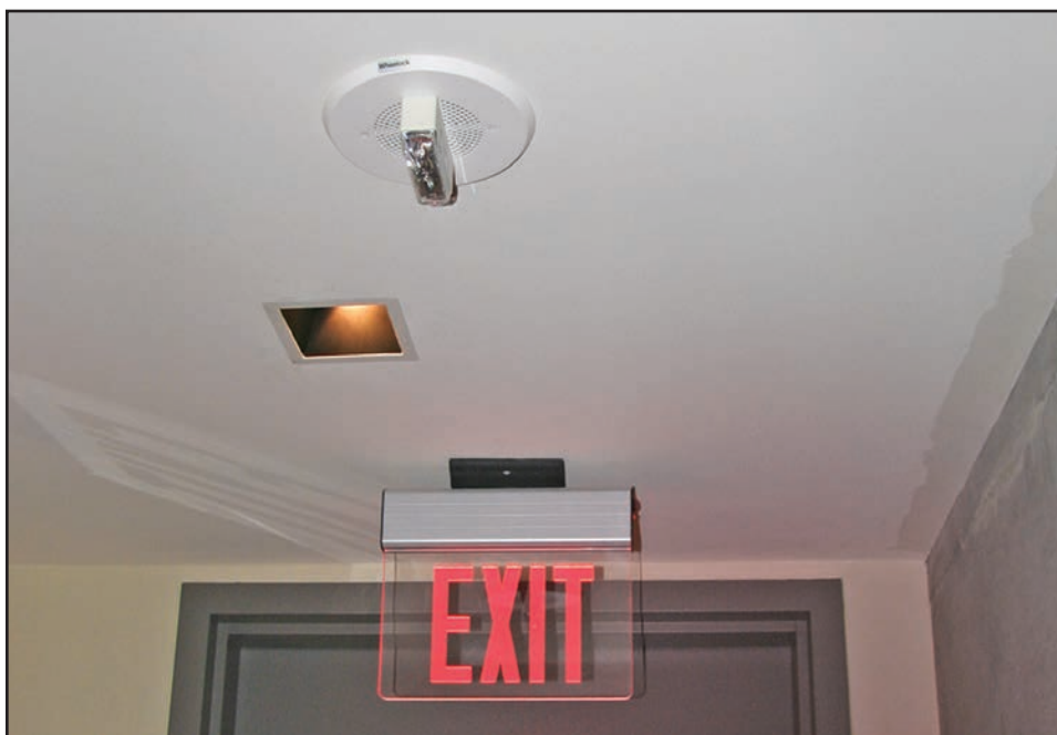
Figure 14.52 The inspector should verify correct placement for visual devices.
