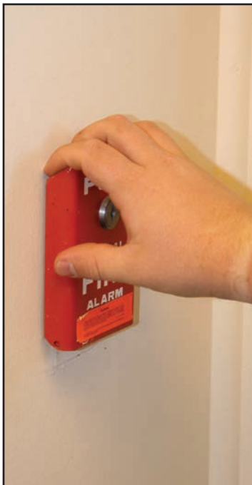
Figure 14.40 Single-action pull stations require only a single motion to trigger an alarm.
