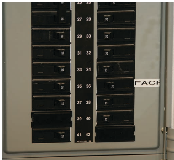
Figure 14.4 On the power supply circuit board, one switch should be permanently labeled as the FACU (sticker in the photo) to ensure that anyone doing maintenance on the circuit board does not deactivate that switch and create a safety hazard.
