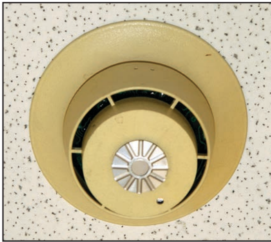
Figure 14.37 A combination heat/smoke detector.
