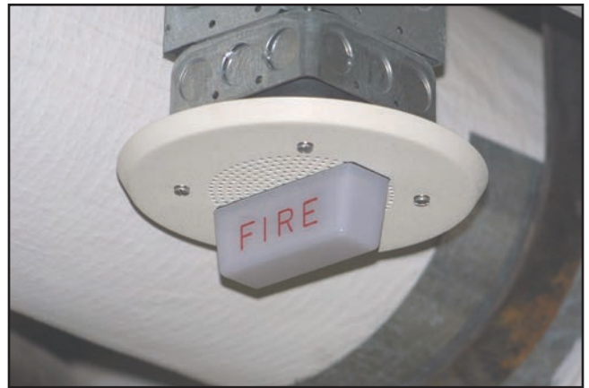
Figure 14.51 Strobe requirements apply to areas that are open to the public. Courtesy of Rich Mahaney.
