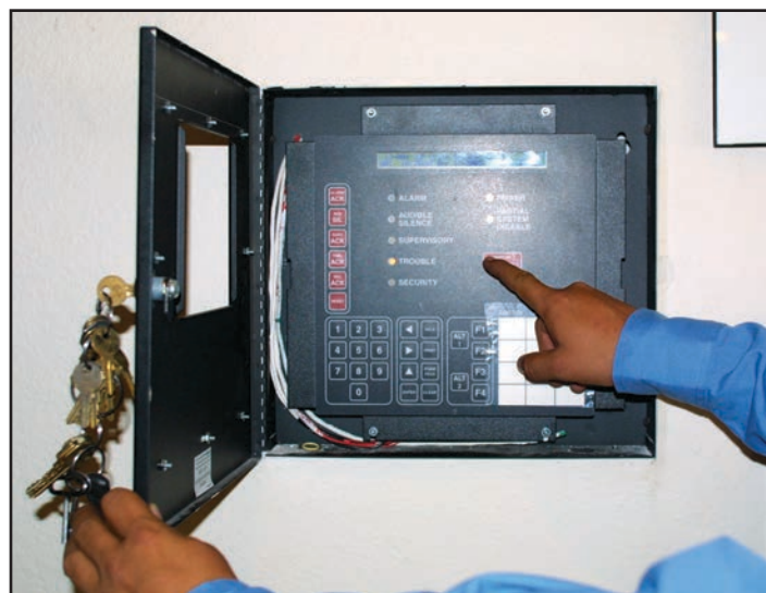
Figure 14.43 Fire department personnel who conduct inspections must have a working knowledge of detection and alarm systems.
