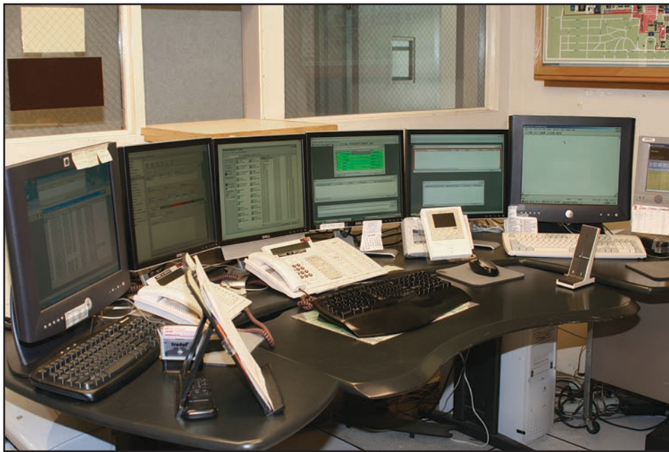
Figure 14.15 Central station receiving sites are housed in an off-site location that receives alarms and routes them to the responding fire department.
