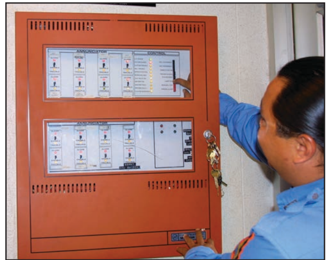
Figure 14.12 Zoned systems are designed to help emergency responders quickly identify the location of a fire.
