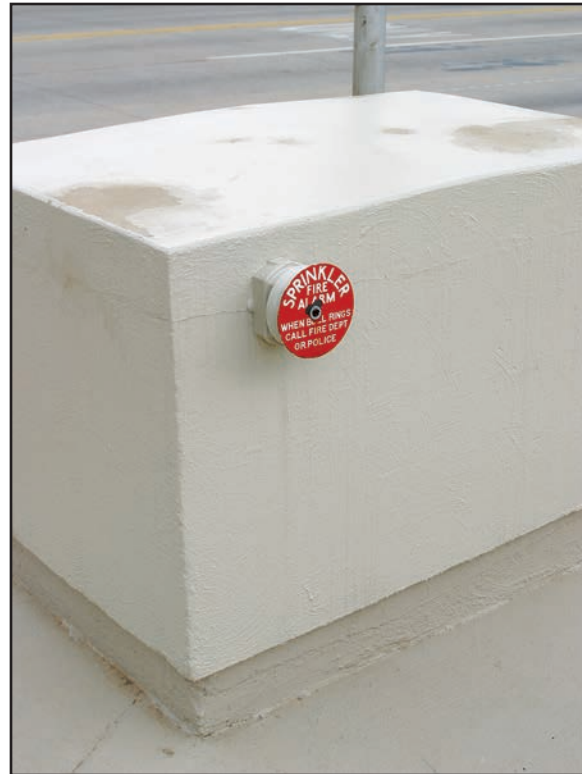
Figure 14.38 A waterflow alarm indicates the flow of water through the system, and may be accompanied by a system drain valve.
