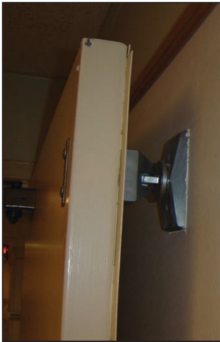
Figure 14.8 Magnetic door closures like this one are designed to remain open during normal building activity and release when alarms are activated to close the door.
