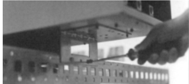
The fusible switch module has a self-aligning bracket screwed to the interior mounting rails.
