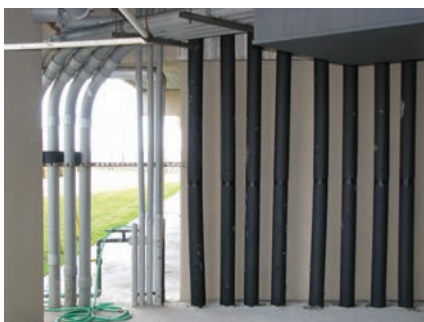
Figure 4-2. Geothermal loop field headers.
