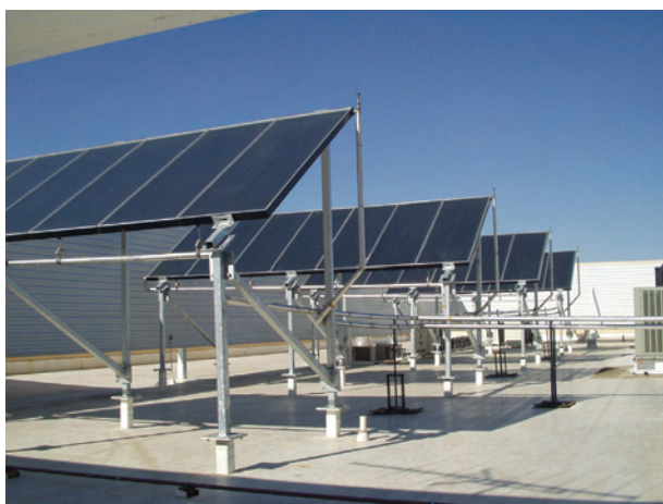
Figure 4-9. Solar panels at the Riverside Medical Clinic.
