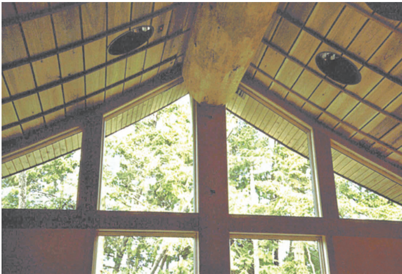
Figure 3-17. Skylights and windows provide an aggregate of twice the already stringent Oregon code standards for energy efficiency.
