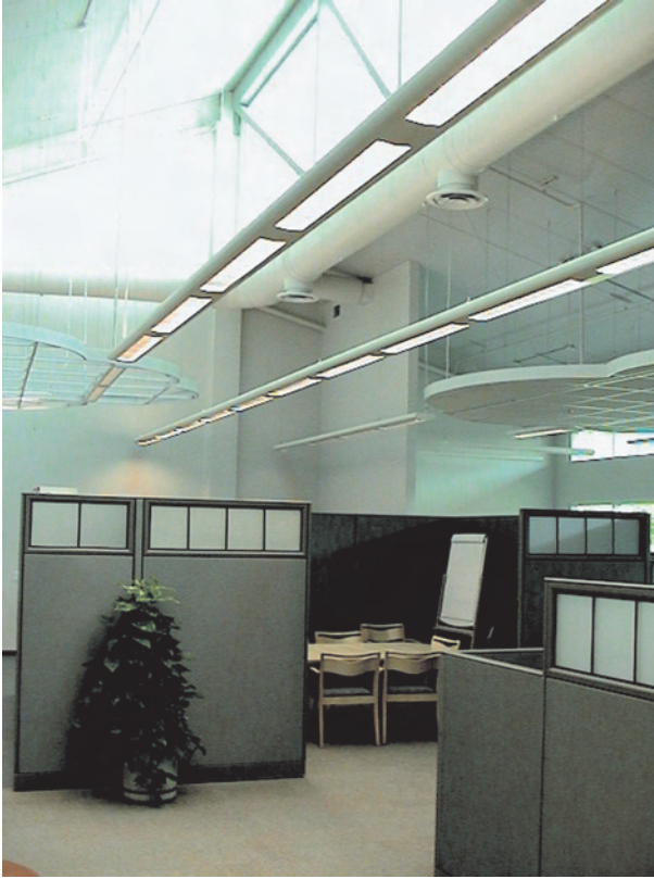
Figure 3-3. A sensor measures the amount of natural light coming in and adjusts overhead fluorescent lights accordingly.
