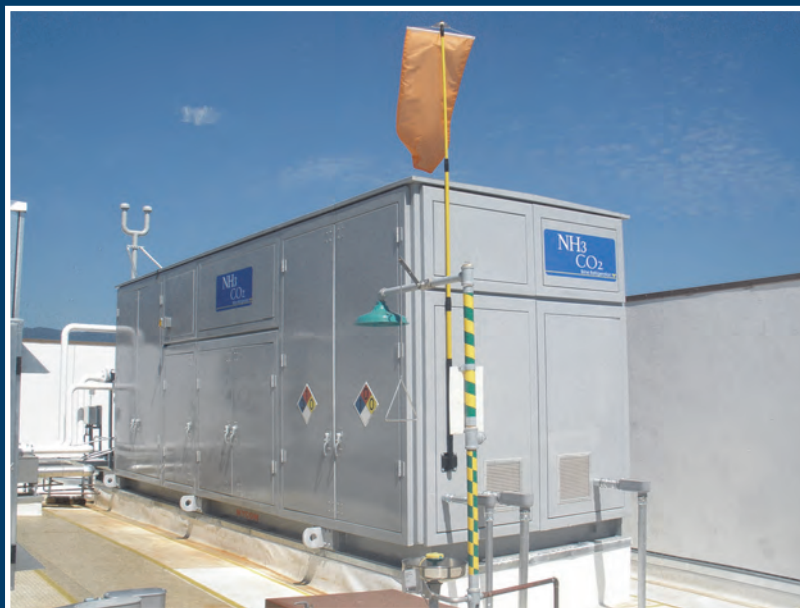
Rooftop Ammonia Refrigeration System Photograph reproduced with permission of CTA, Inc.
