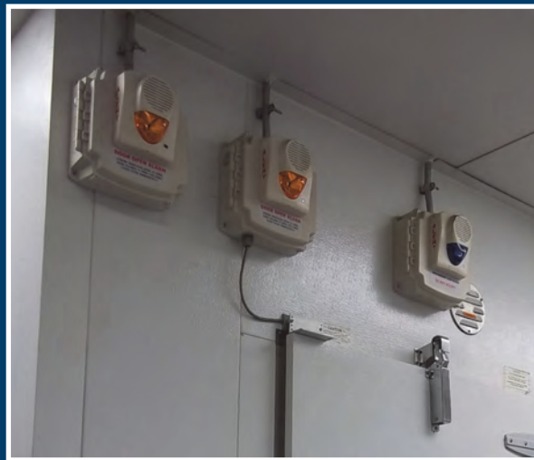
Horn and Strobe Door Alarms (left and center) and Leak-Detection Strobe Alarm (right)
