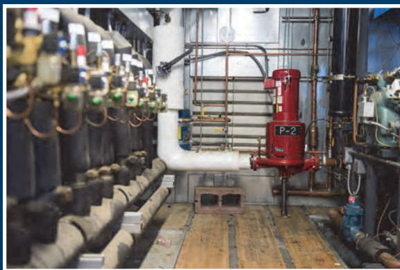
Waste Heat Recovery System Glycol Pump
