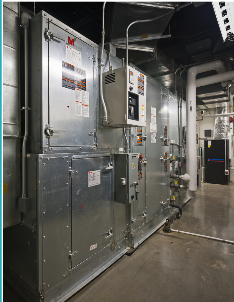
Outdoor Air-Handling Units
