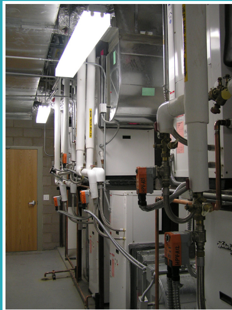
Geexchange Heat Pumps
