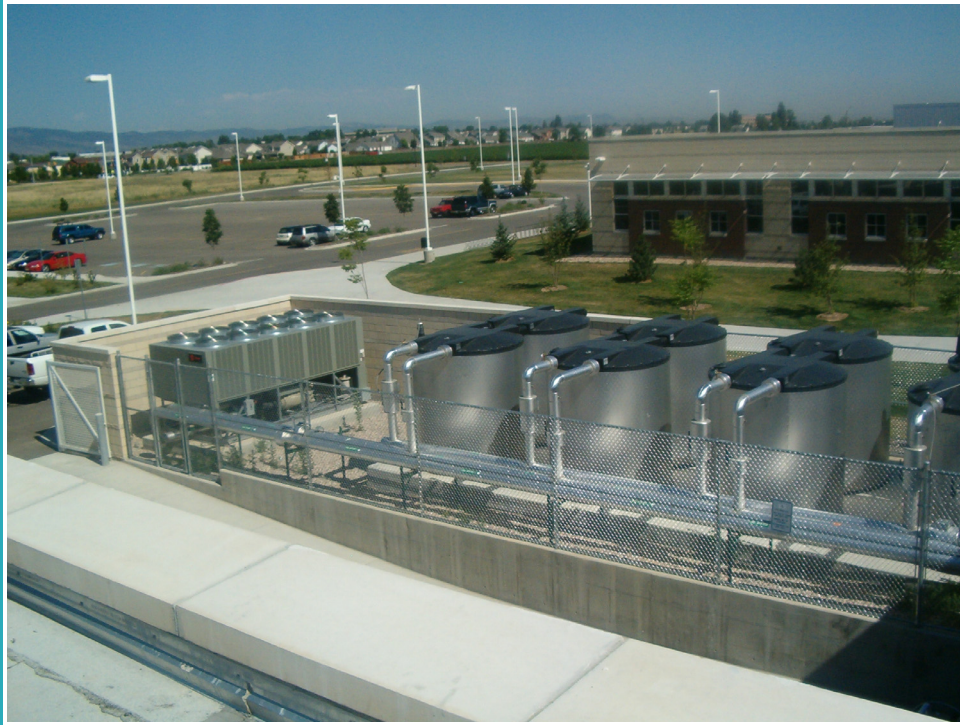
Ice Storage Tanks and Air-Cooled Chiller
