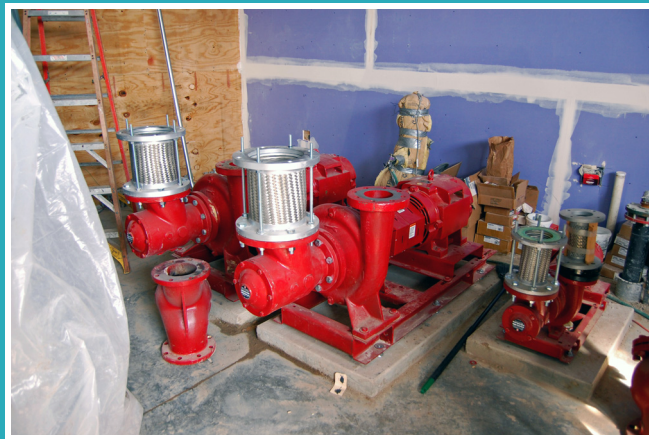
Pump for Closed Loop Hybrid Heat Pump System Source: Greensburg GreensTown (courtesy of DOE/NREL)
