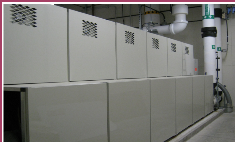
Energy Recovery Chiller System Photo courtesy of KJWW Engineering
