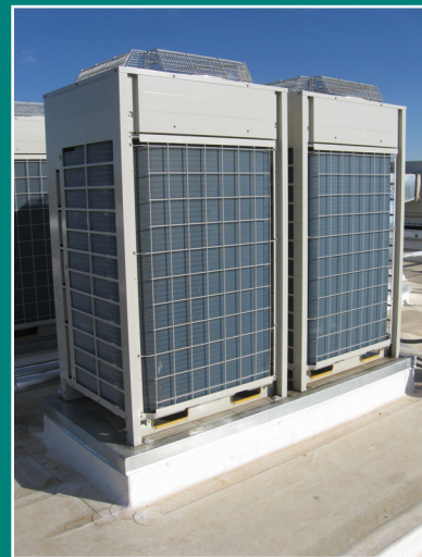
VRF HVAC System on Roof
