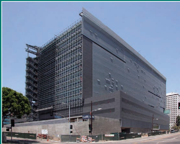
Armature for PV Panels Source: Arup
