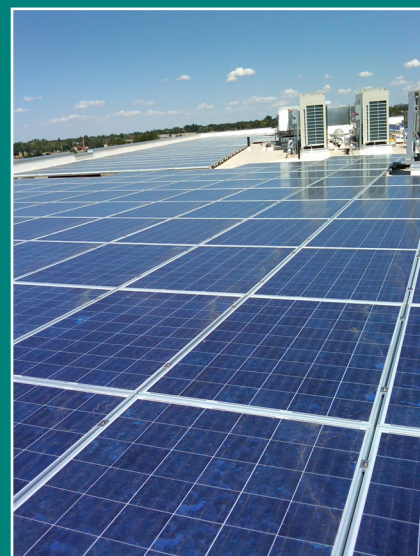
Roof PV Panels
